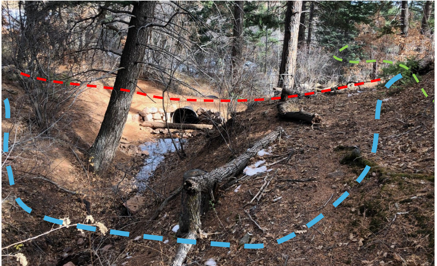
AN7 With remove and relocation of 36" culvert. Hiking only trail E9 on the right of image
