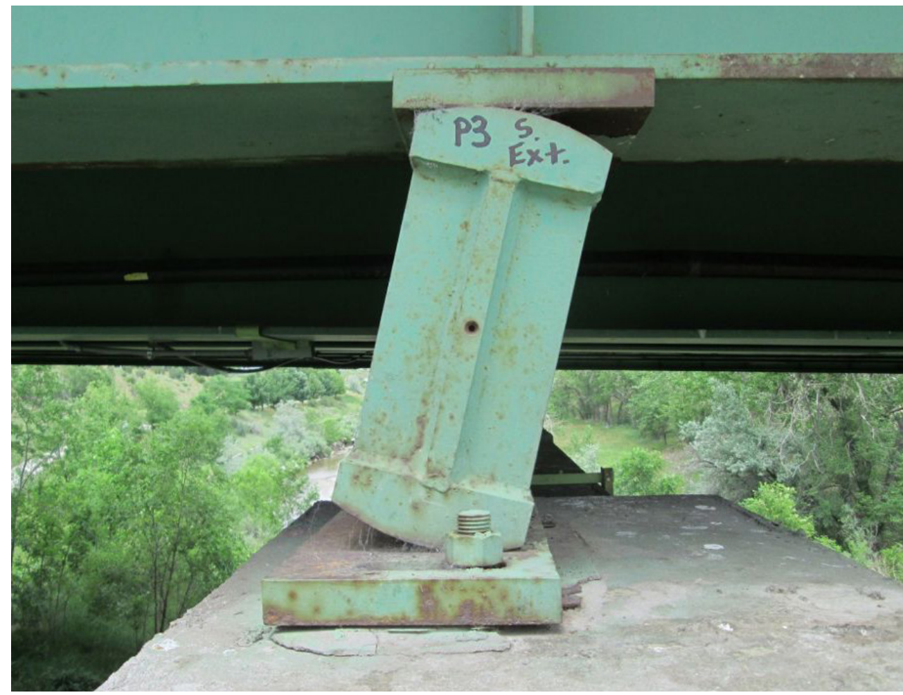
Tilted Girder Bearings Past Critical Angle
