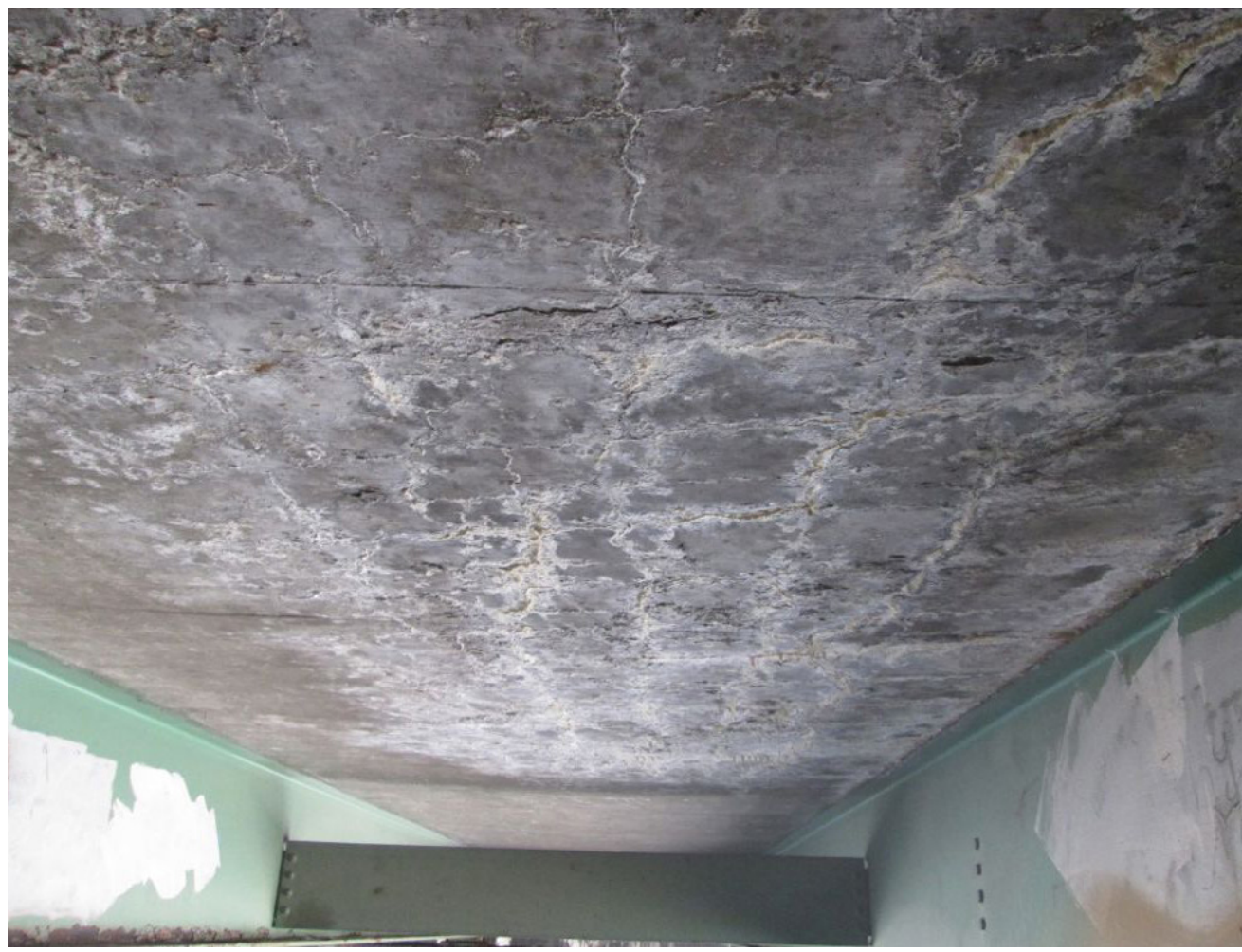
Spalling and Cracking Deck
