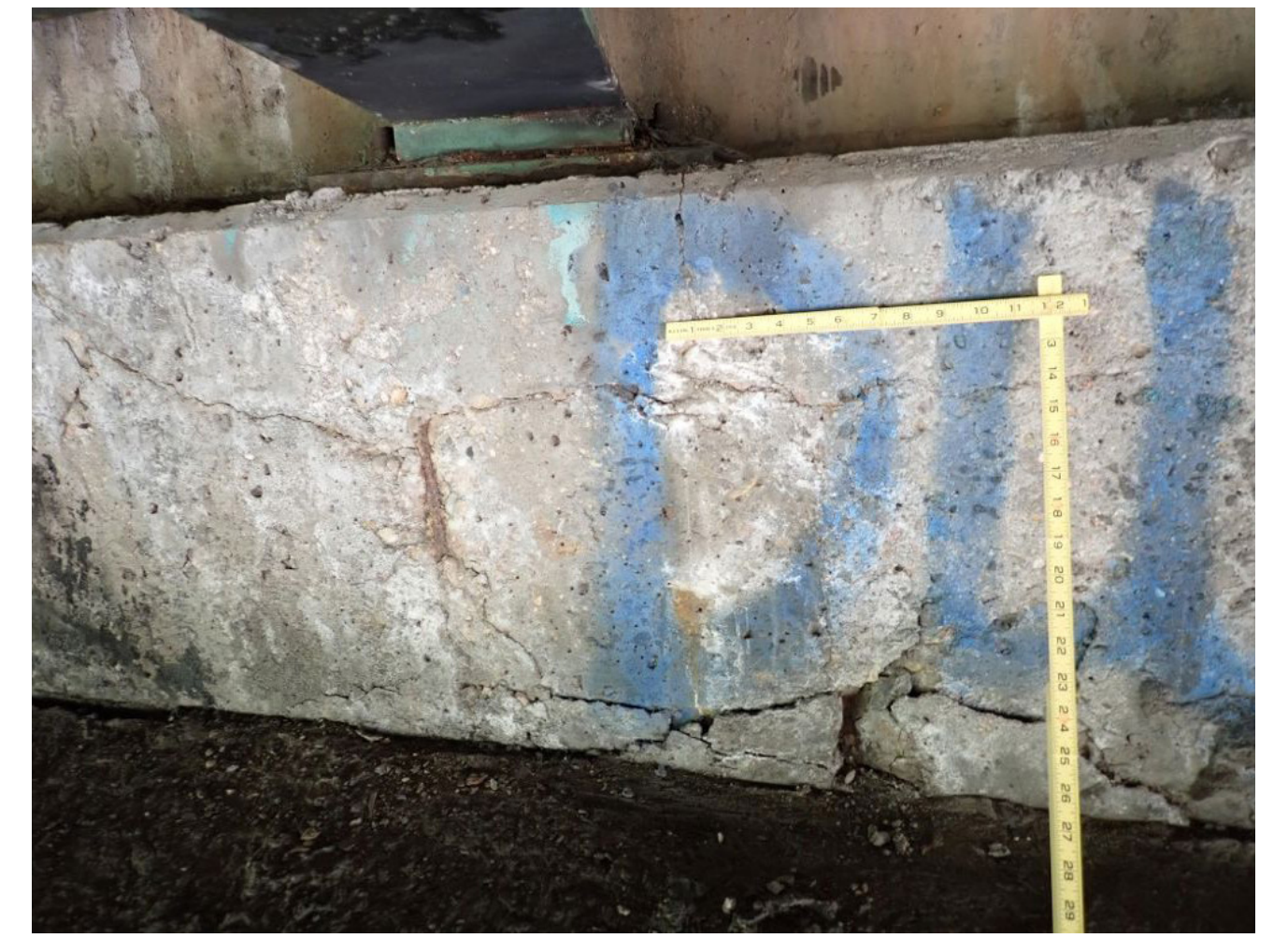
Cracked and Spalled Substructures
