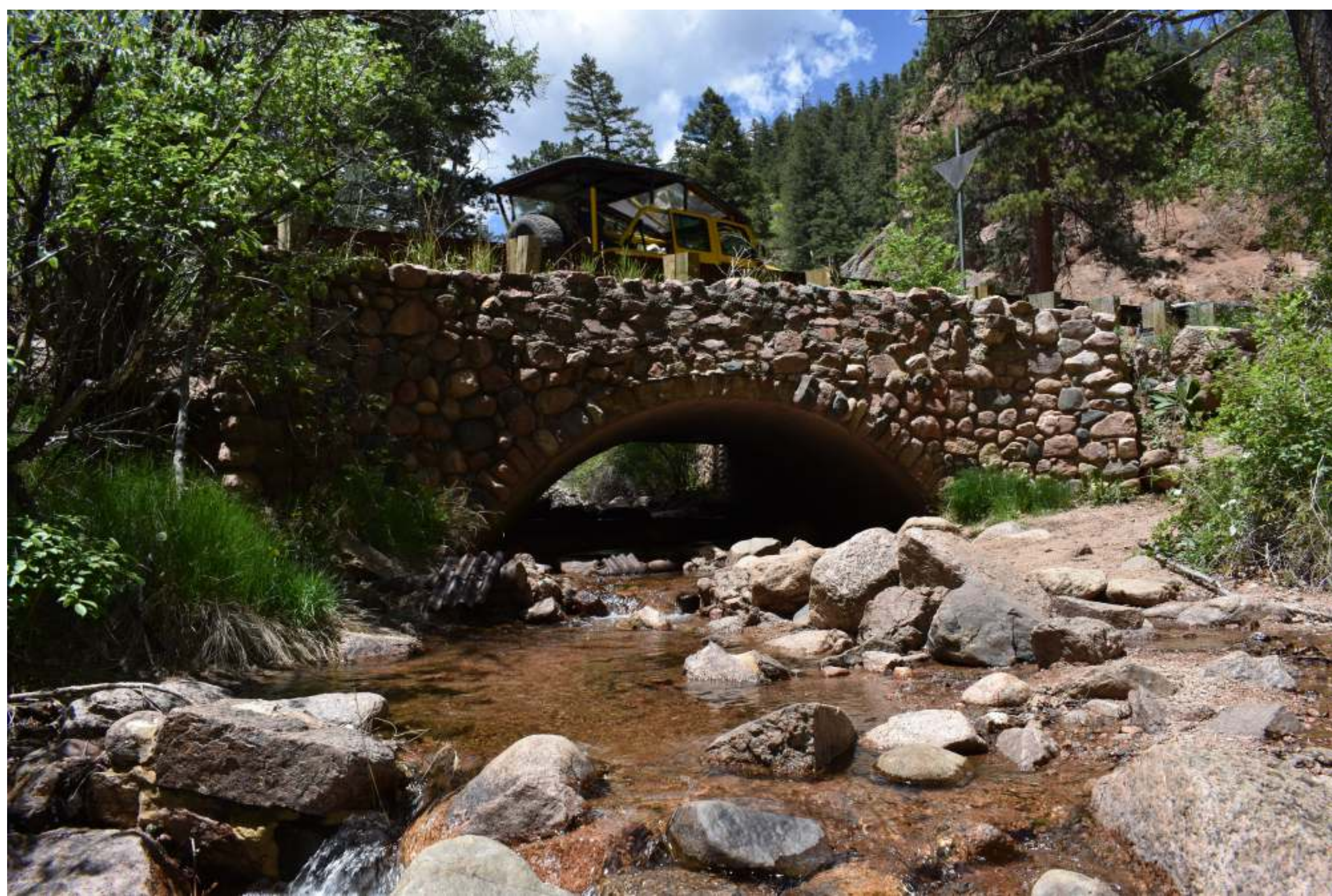
This bridge is a "contributing feature" of North Cheyenne Cañon Park and North Cheyenne Cañon Road because it retains aspects of its original 1920s design. CDOT and the Corps will consult with the SHPO on the effects of replacement pursuant to Section 106 of the NHPA.
